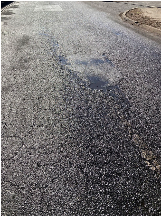
S4 road (before). Typical surface condition
